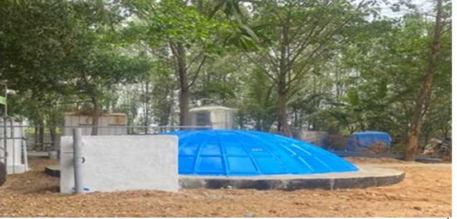
TAPF: Biogas Plant and TAPF Kitchen at Kandi Telangana
